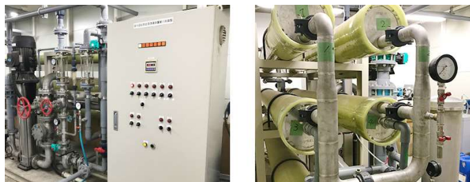
Reverse Osmosis (RO) Filtration Equipment
