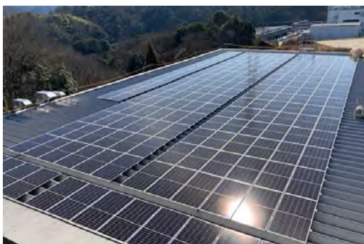
Solar panels installed at the Salad Club Mihara Plant
