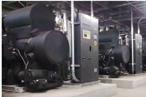
Ammonia freezer units
