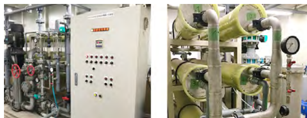
Reverse Osmosis (RO) Filtration Equipment
