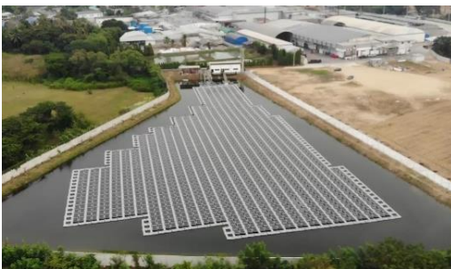
Solar panels installed on the surface of the reservoir on the premises of the Kewpie Thailand Plant
